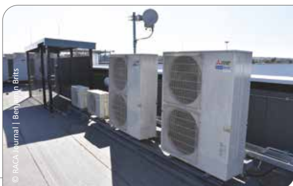
DX condensers (for one of the server rooms).
