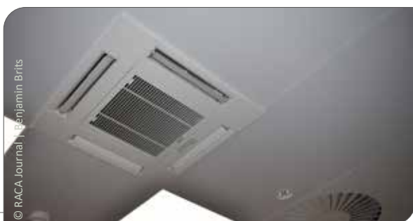
An example of the ducted cassette units and diffusers located in one of the wards of the hospital.
