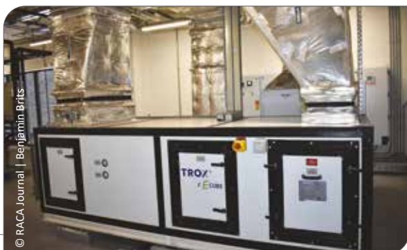
One of the VRF theatre air handling units.
