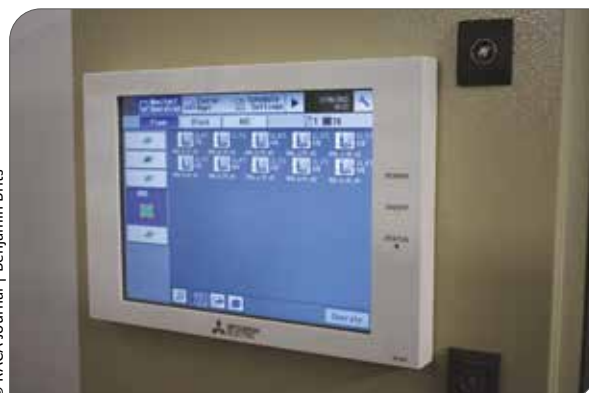
VRF central controller.
