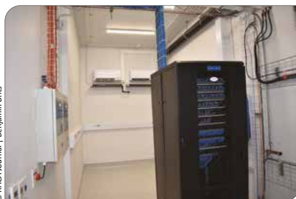
One of the de-centralised server rooms. Each room at the site is serviced with either DX or VRF units based on room positioning.
