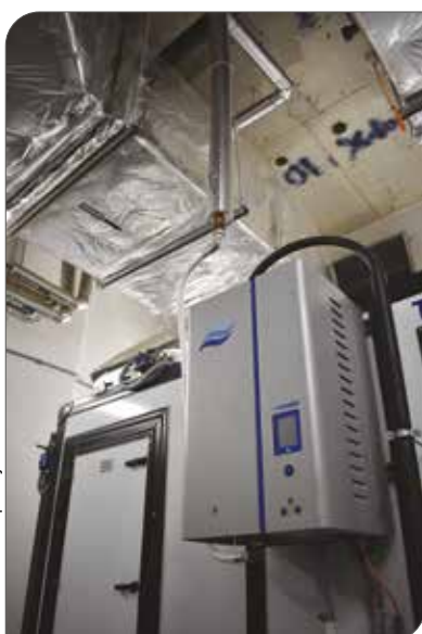
A theatre AHU humidifier.
