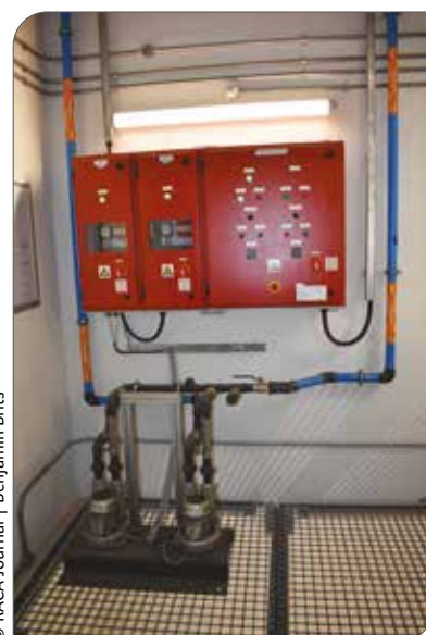
The anaesthetic gas scavenging system.
