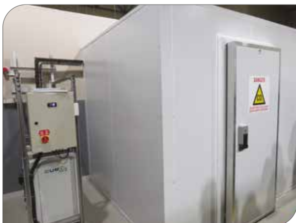
A life size cold room with a CO 2 system for the training in natural refrigerants.
