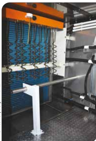
Internal view - AHU (DX coil, electric heater bank and humidifier).
