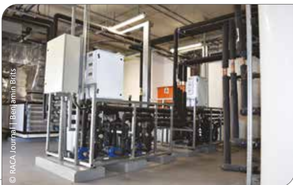
A decentralised heat recovery hot water plant.
