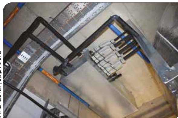
One of the VRF control box.
