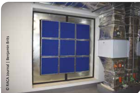
One of the fresh air intakes for the main plantroom located on the roof.
