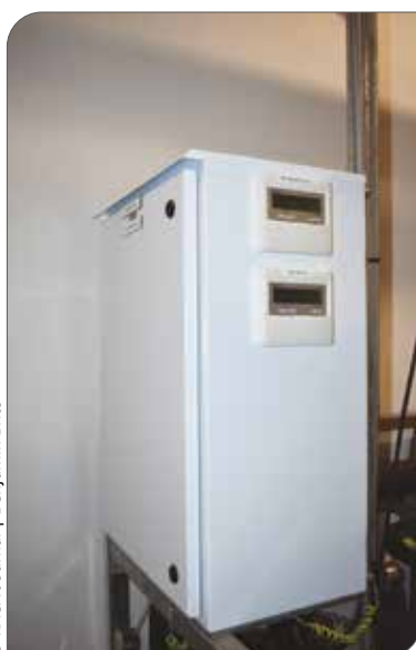
One of the MCC panels.
