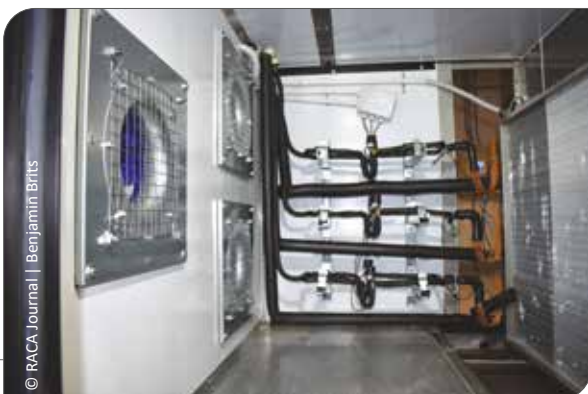
Internal view - AHU (fan and LEV kits).
