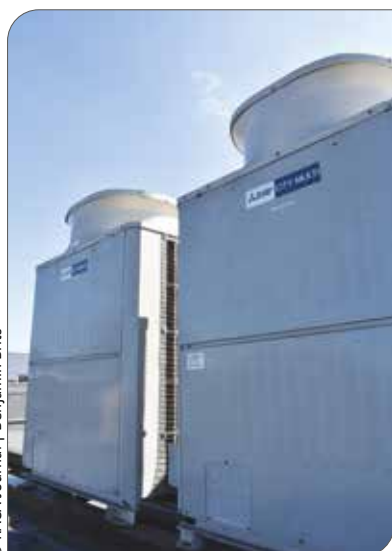
Some of the heat recovery condensers located on the roof.
