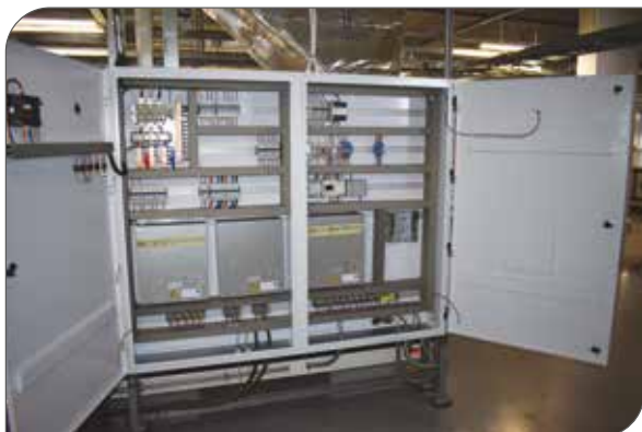
Internal view - AHU (MCC).
