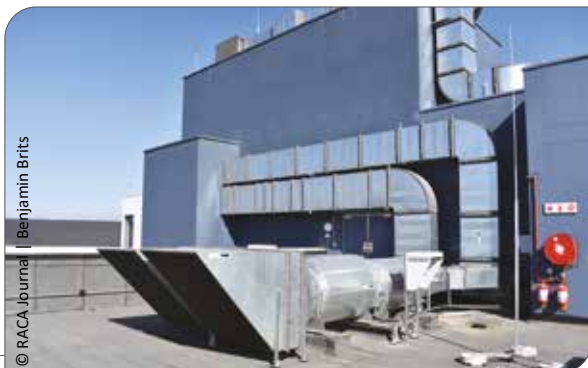
The energy centre fresh air system.
