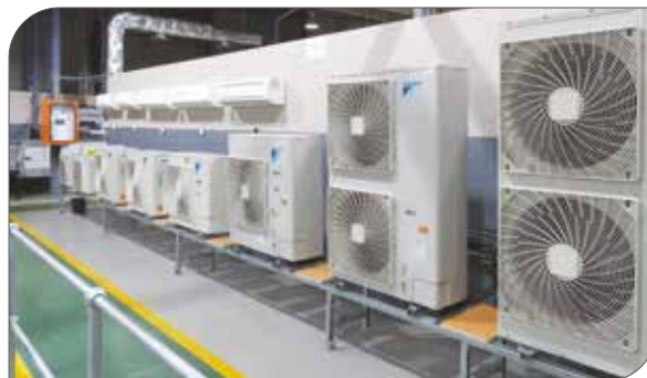
A Variety of different air conditioning systems are used in the training of skills for the A/C industry.
