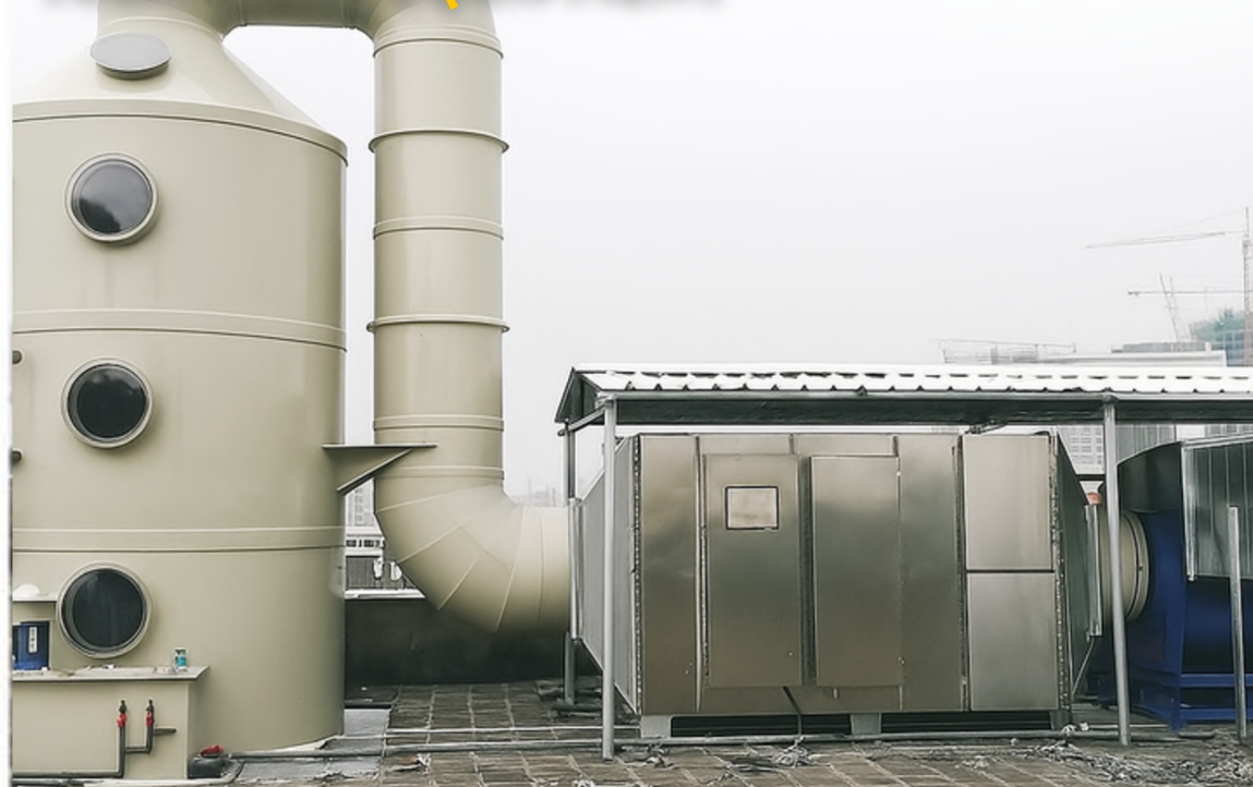
EXHAUST GAS TREATMENT EQUIPMENT
