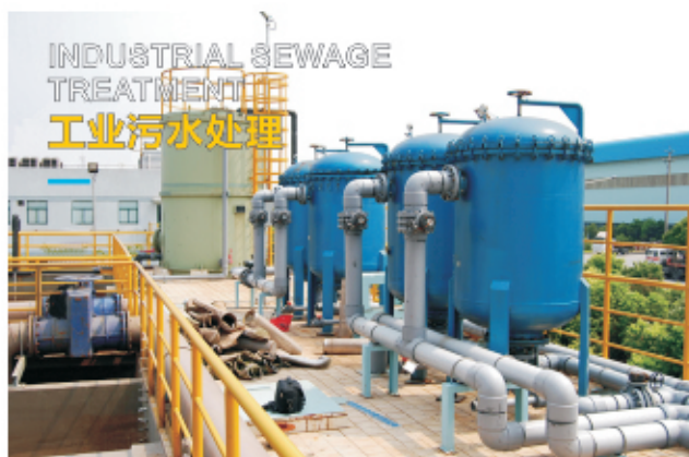
ULTRAFILTRATION EQUIPMENT 超滤设备
