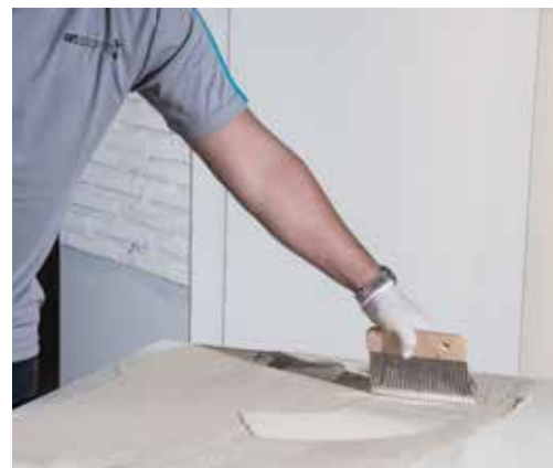
4. The prepared mixture is distributed evenly behind the panel with the help of a 3 mm metal comb.
