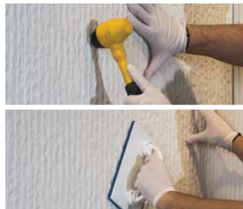
5. The panel is mounted on the wall, and the assembly process is completed with the help of a plastic hammer and sponge trowel to ensure it is firmly fixed.
