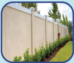
Compound Wall for Entire Layout
