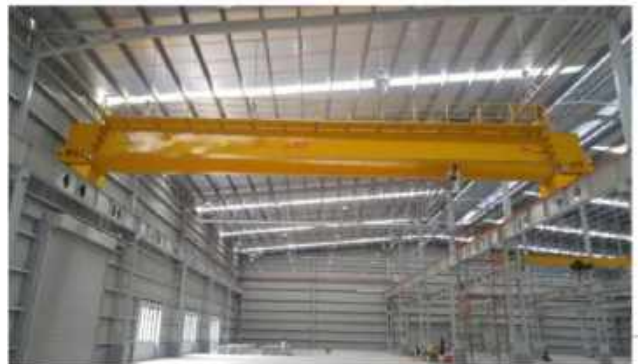
PAWELL DOUBLE GIRDER OVERHEAD CRANE CAP 15 TON X 20Meter SPAN x 70Meter Long Travel ( 1UNIT )
