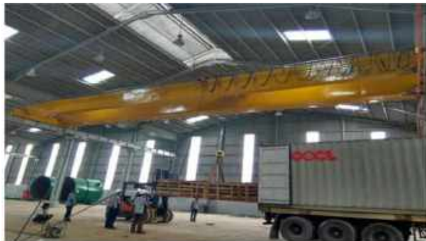
PAWELL DOUBLE GIRDER Overhead CRANE CAP 12 TON X 21 Meter SPAN x 70Meter Long Travel ( 3UNIT )
