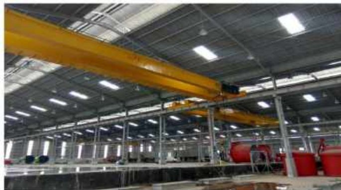
PAWELL DOUBLE GIRDER Overhead CRANE CAP 7TON X 20Meter SPAN x 215Meter Long Travel ( 3UNIT )
