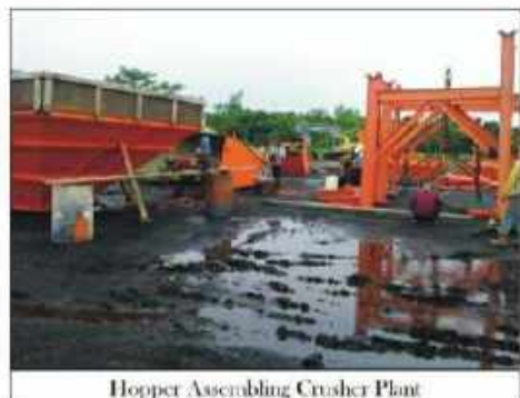
Hopper Assembling Crusher Plant
