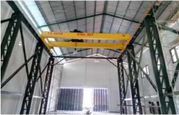
PAWELL DOUBLE GIRDER OVERHEAD CRANE CAP 32TON X 12Meter SPAN x 20Meter Long Travel ( 1UNIT )
