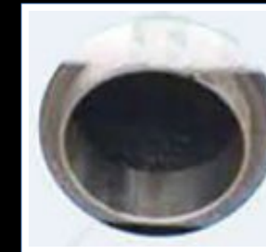
Sewage Drainage Exit Pipe
