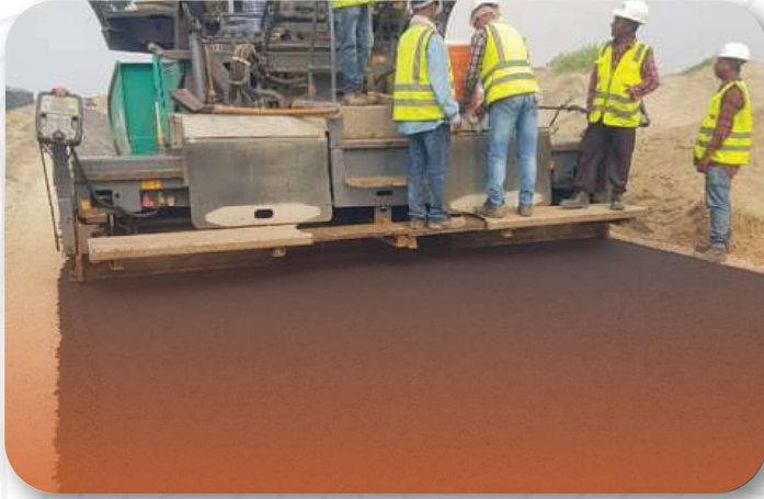
Riyadh Ind City Road Works We're bringing our expertise to Riyadh, the 2034 FIFA World Cup host, by paving 42 Km of local Roads.
