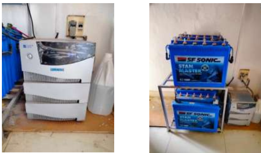
Figure 2: Existing inverter and battery pack
